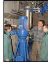
Allweiler sludge pump
